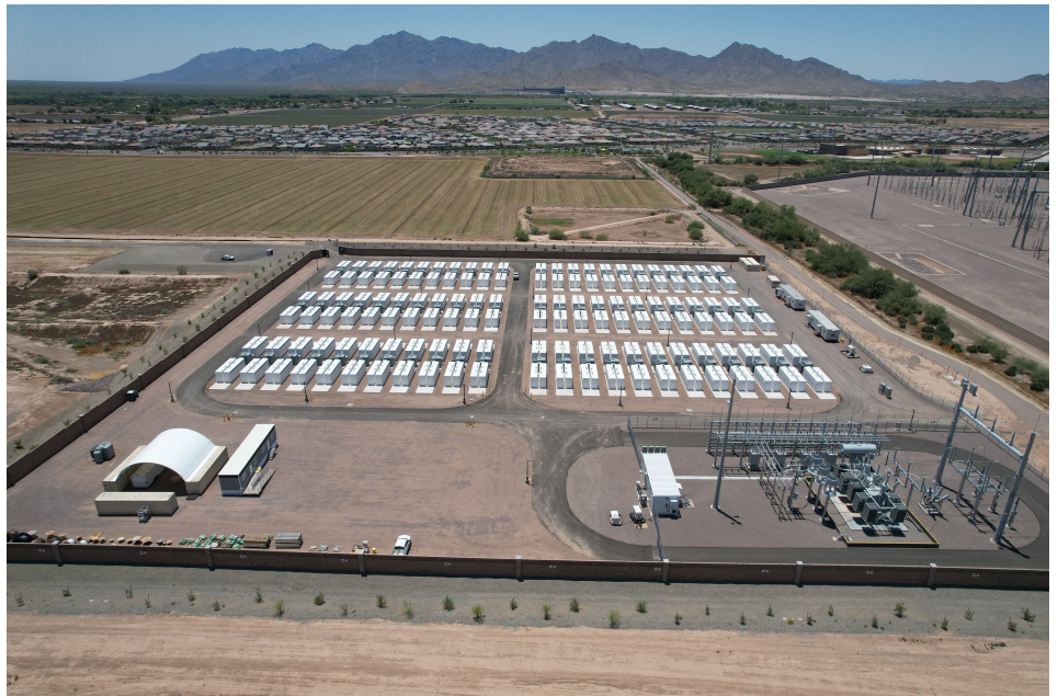
Plus Power's Sierra Estrella Energy Storage facility (image courtesy of Plus Power)
